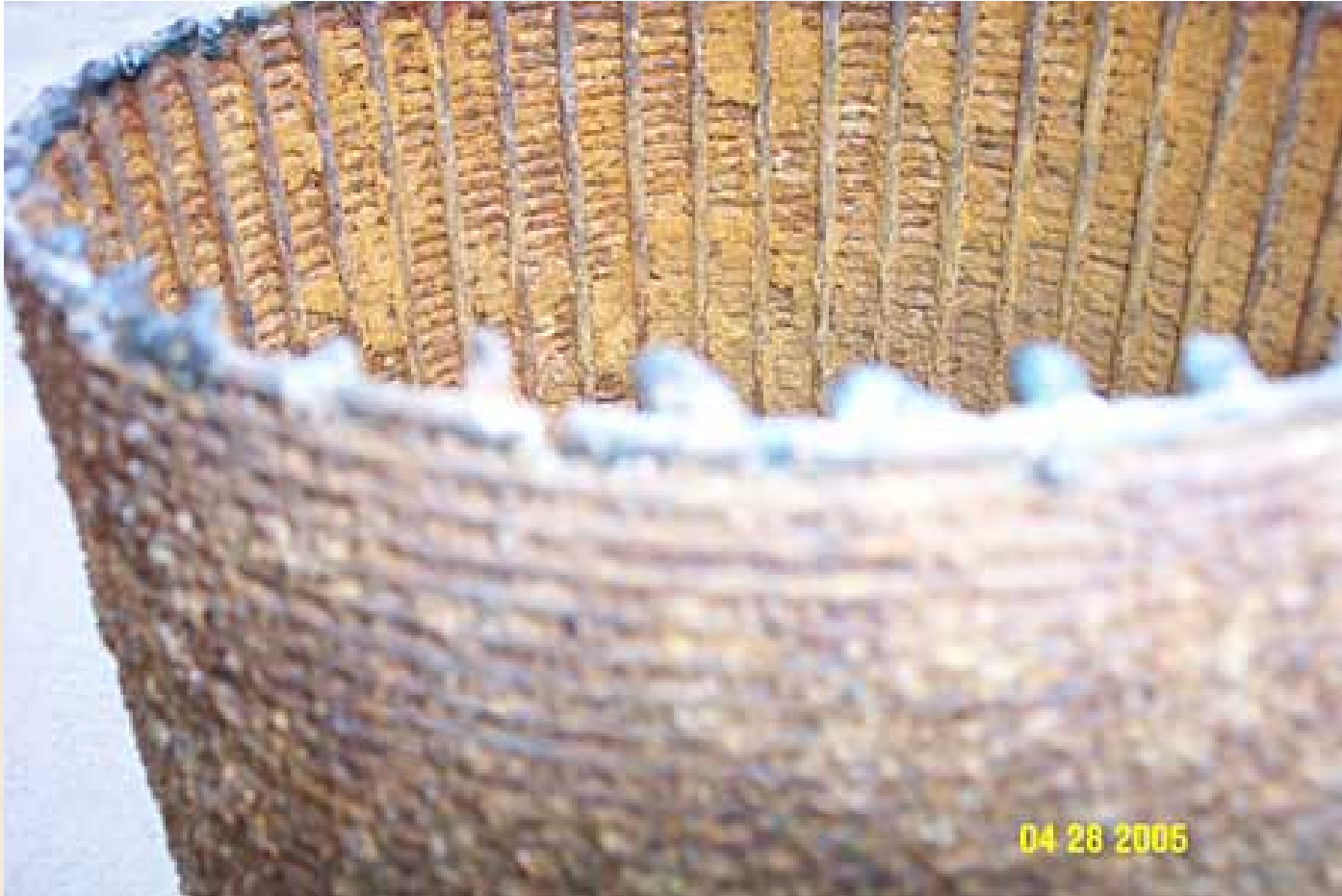
Figure 3: Encrusted minerals on the inside of a totally plugged well screen
